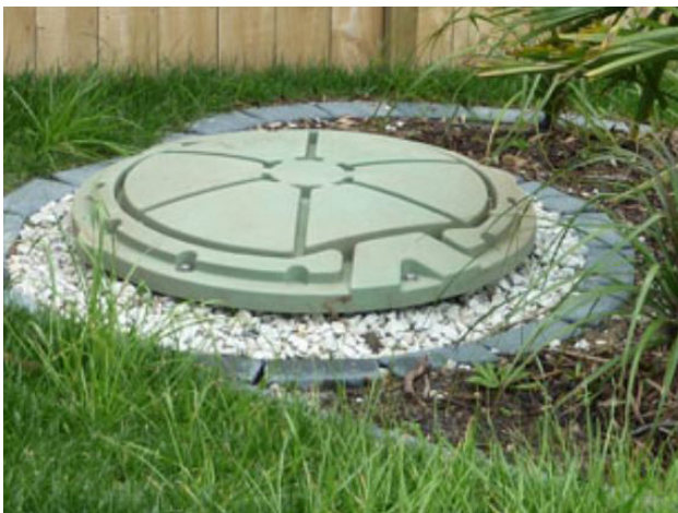
What the tank looks like installed, with just the lid visible at ground level.
