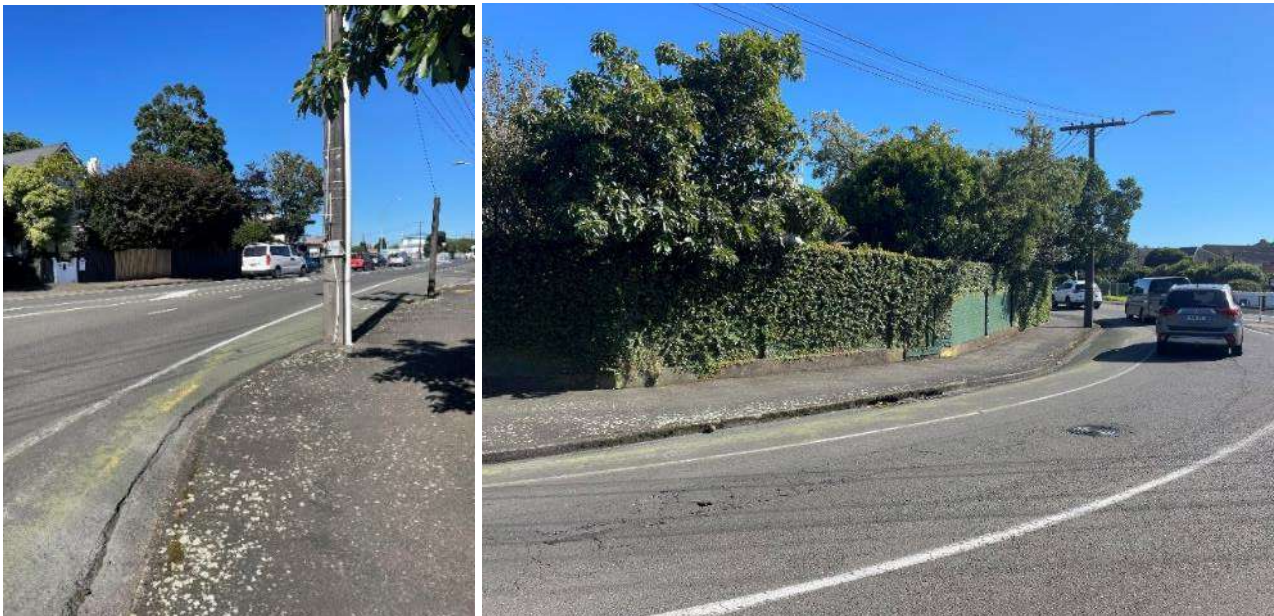
Figure 4-33: Narrow cycleway with fading markings at intersection of Tukapa St and Morley St
