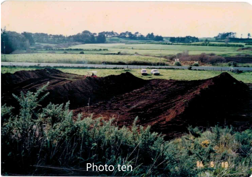
Range 5 and 6 under development in May 1984. We can see State Highway 3 and the entry gate behind the cars.
