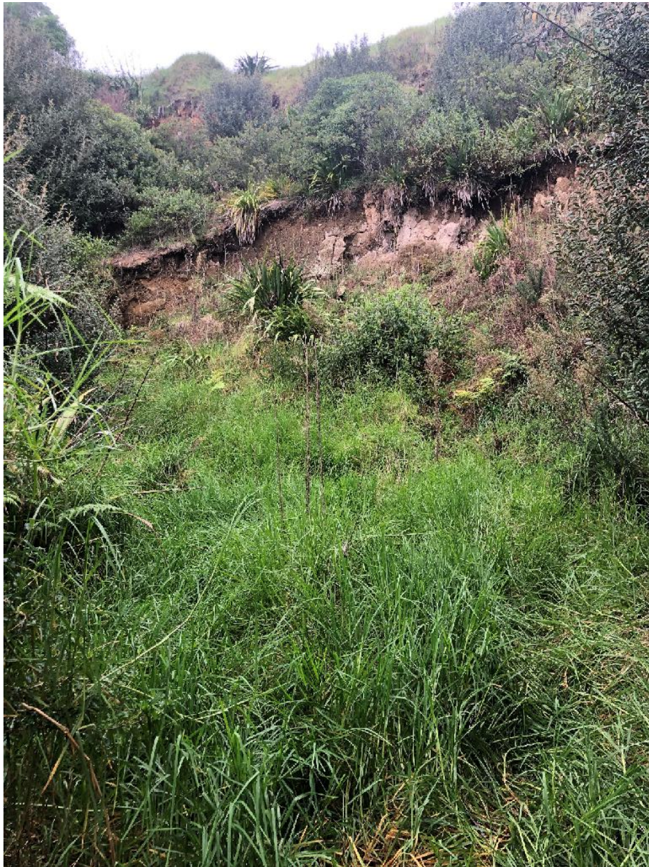
Photo 1: view from base of slip looking up to the top of the slope.
