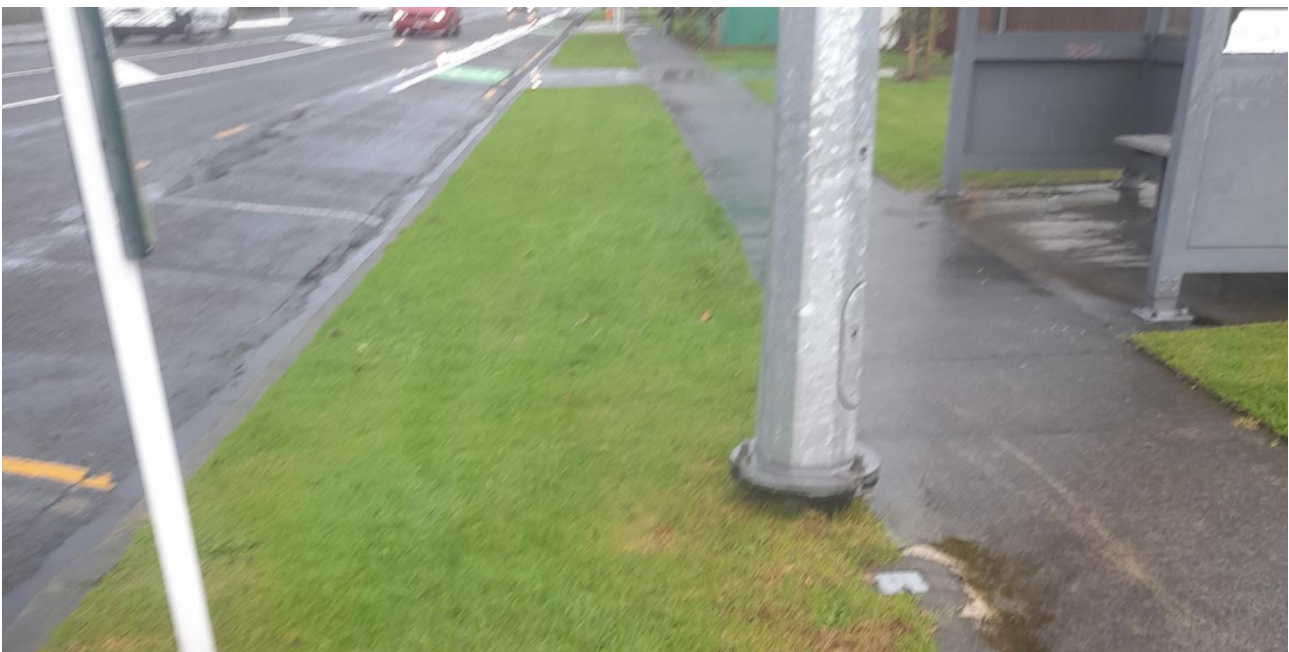
Figure 5-2: Bus stop with no footpath to bus connection.
