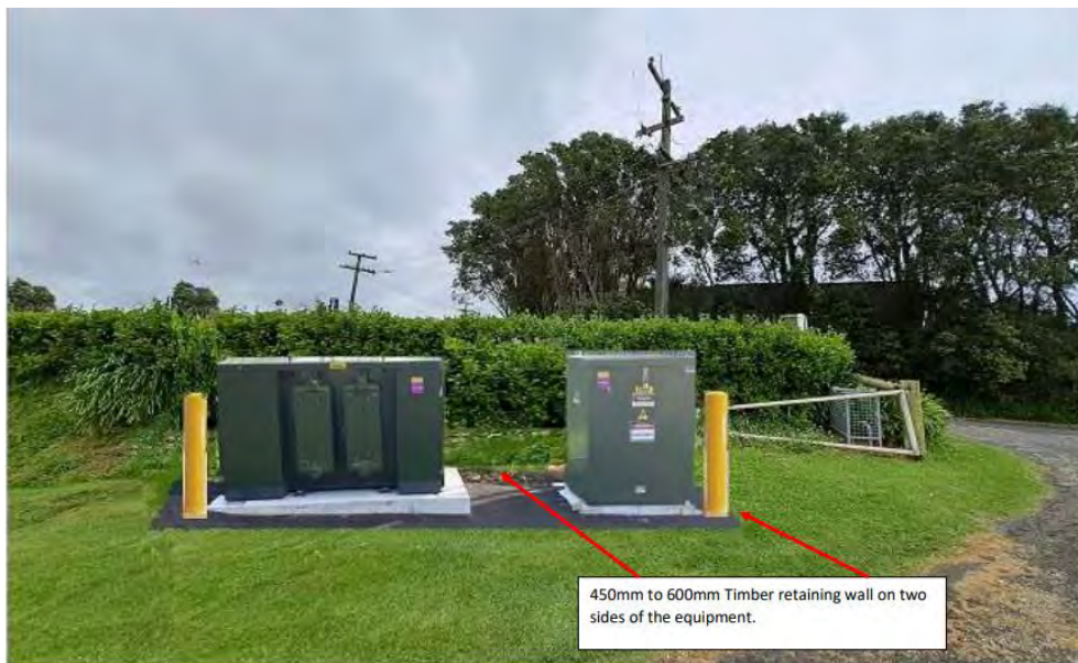
Indicative position of 500kVa Ground Mount transformer and Switchgear. Protective bollards positioned each side of equipment to protect against vehicles. Asphalt around the base of the equipment.
