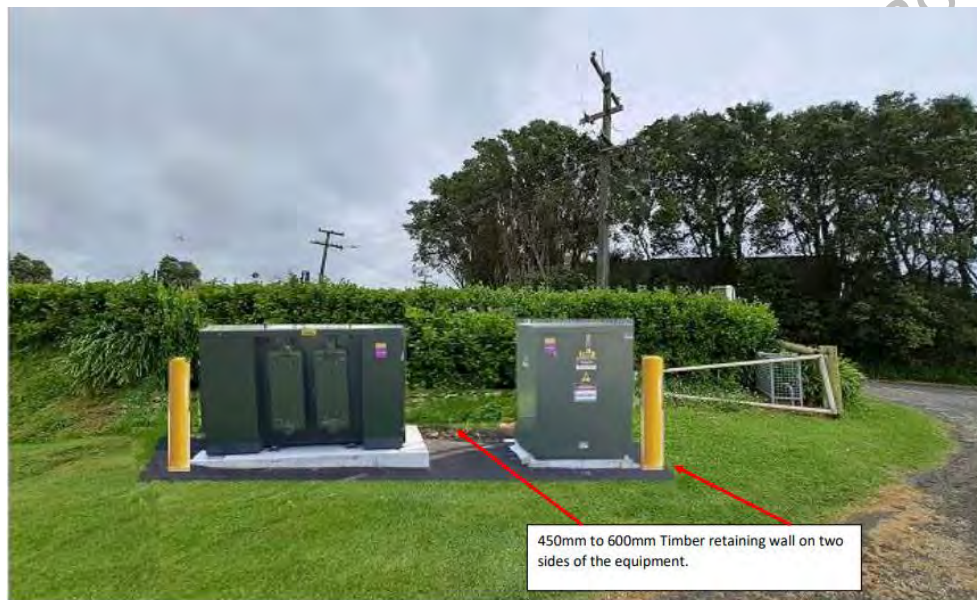
Indicative position of 500kVa Ground Mount transformer and Switchgear. Protective bollards positioned each side of equipment to protect against vehicles. Asphalt around the base of the equipment.
