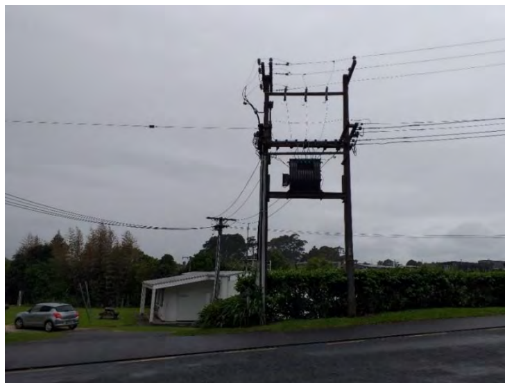
Figure 1: Current H Structure Transformer Pole – Jans Terrace, identified for removal.
