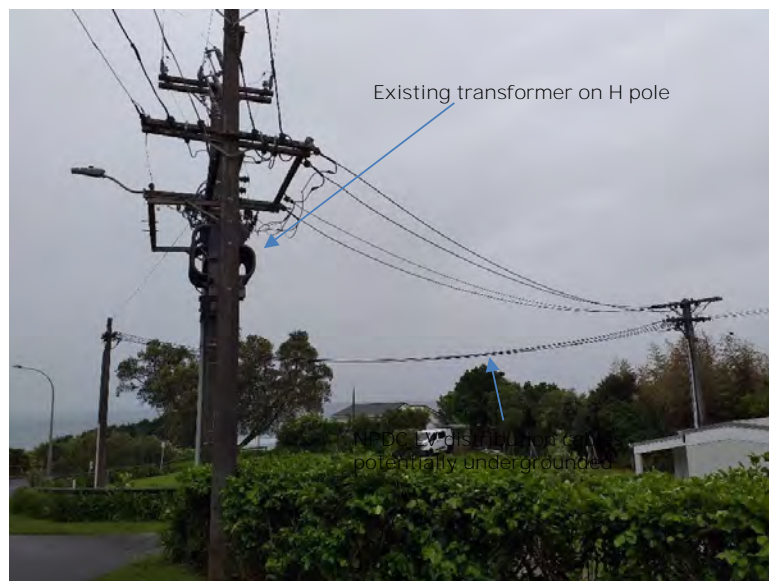
Figure 3: Pole Mounted transformer and NPDC owned LV Distribution cables into Campground
